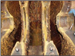
Corroded pump volute
